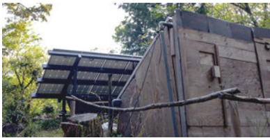
Solar battery panels powering the on-site equipment
