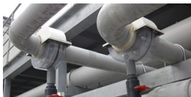
Double joints in piping Monitoring and prevention of liquid leakages
