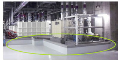
Drainage dike Prevents wastewater from leaking underground or into public water areas.
