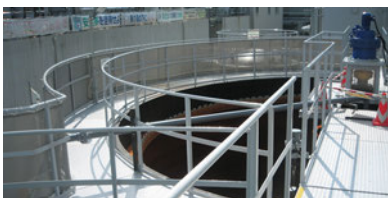
Wastewater treatment Stable processing system that prevents discharge of wastewater
