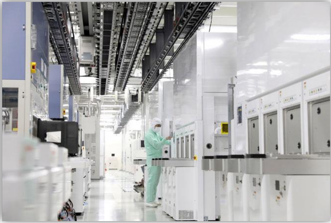
The clean room of Fab7, Yokkaichi Plant
