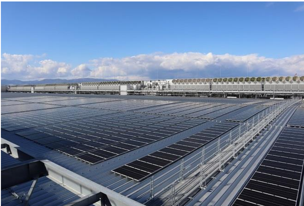
Photo caption: Solar panels on Kitakami Plant Fab 1 roof
